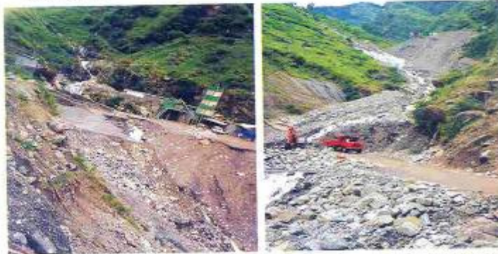
Fig. 30. View of the slope instabilities in the Dhauliganga project area, Distt. Pithoragarh (U.A.)
