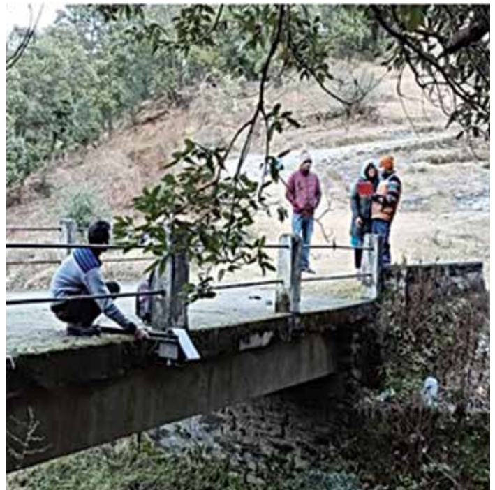
Fig. 4: Installation of water level recorder in Devalikhan recharge zone
